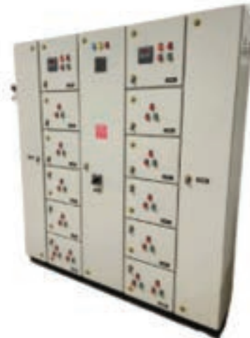
MCC (Motor Control Centre) Panel
