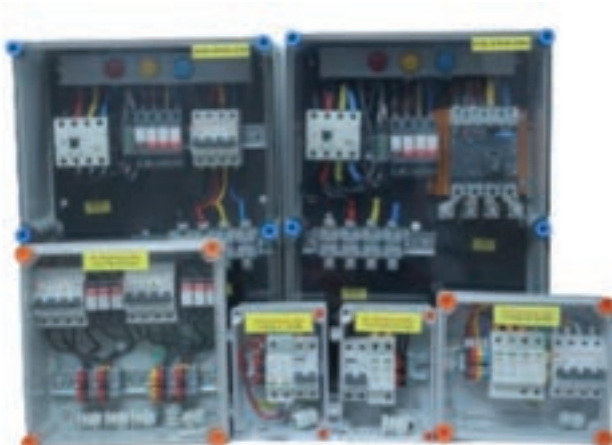
Solar ACDB/DCDB Box
